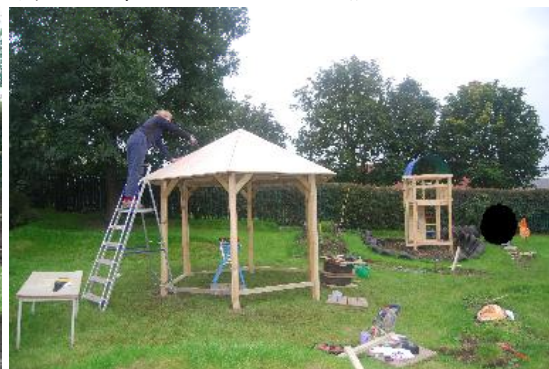
A gazebo was built in the centre of the area and a tower above a sandpit to one side. See Chris up the ladder!
